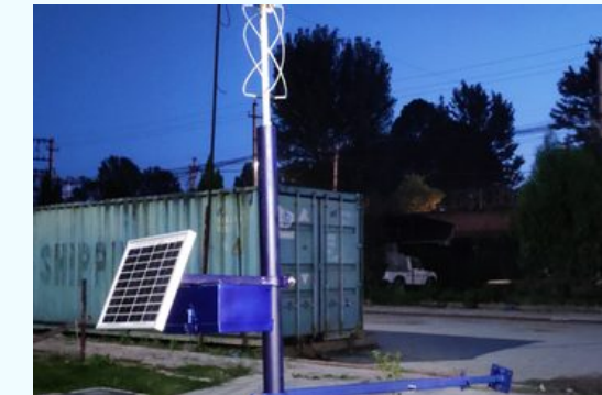
Ground Station Terminals
